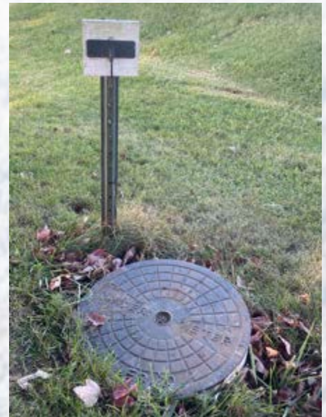
Properly placed lid on top of meter pit.
