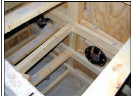
Pipes in Trench Drain
